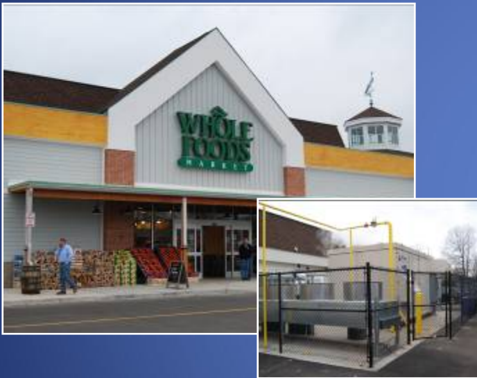
200 kW UTC Power Fuel Cell
