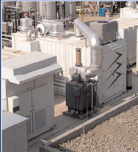
900 kW FuelCell Energy Fuel Cell
